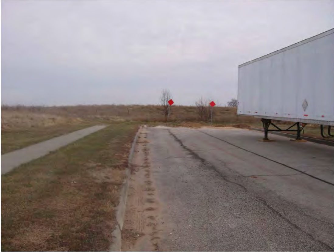
Photo 2 – View of the dead-end at northern portion of NE 104 th Street just north of the Eagle Drive intersection. Road and pedestrian infrastructure abruptly ends at this location. Photo looking north.
