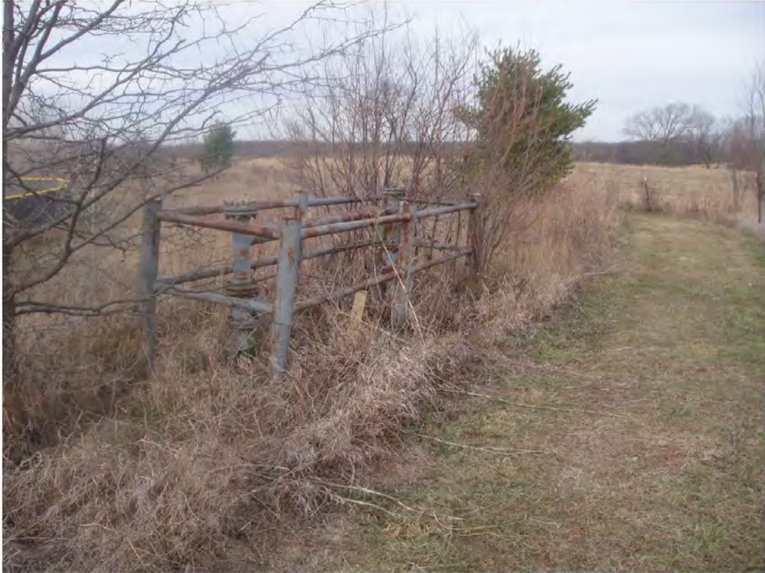
Photo 5 – Gas pipeline relief valve located just south of the north central portion of the proposed Redevelopment Area. Immediately adjacent to the right of this location the gas line moves north through the Redevelopment Area. Photo looking west.
