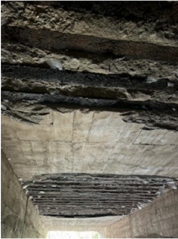
Figure 4 – Excessive Spalling within Box Culvert
