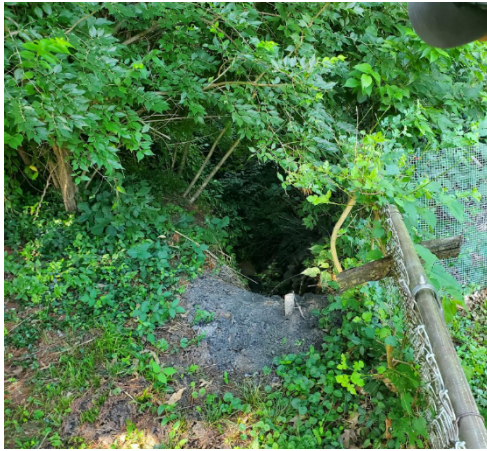
Figure 2 – Creek Eroding Into Private Property
