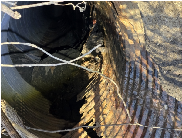
Figure 3 - 54" Corrugated Metal Pipe Outfall Before Project
