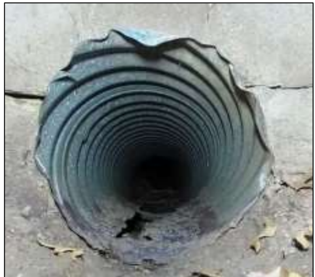
A23-24-890: Pipe rusted through at the bottom
