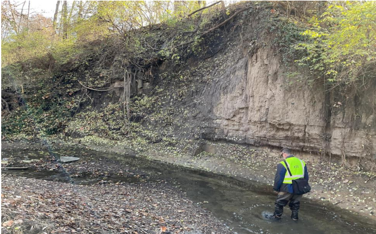
Figure 2-8. Bank Failure Observed on Stream 7 (Location ID: S7.66)
