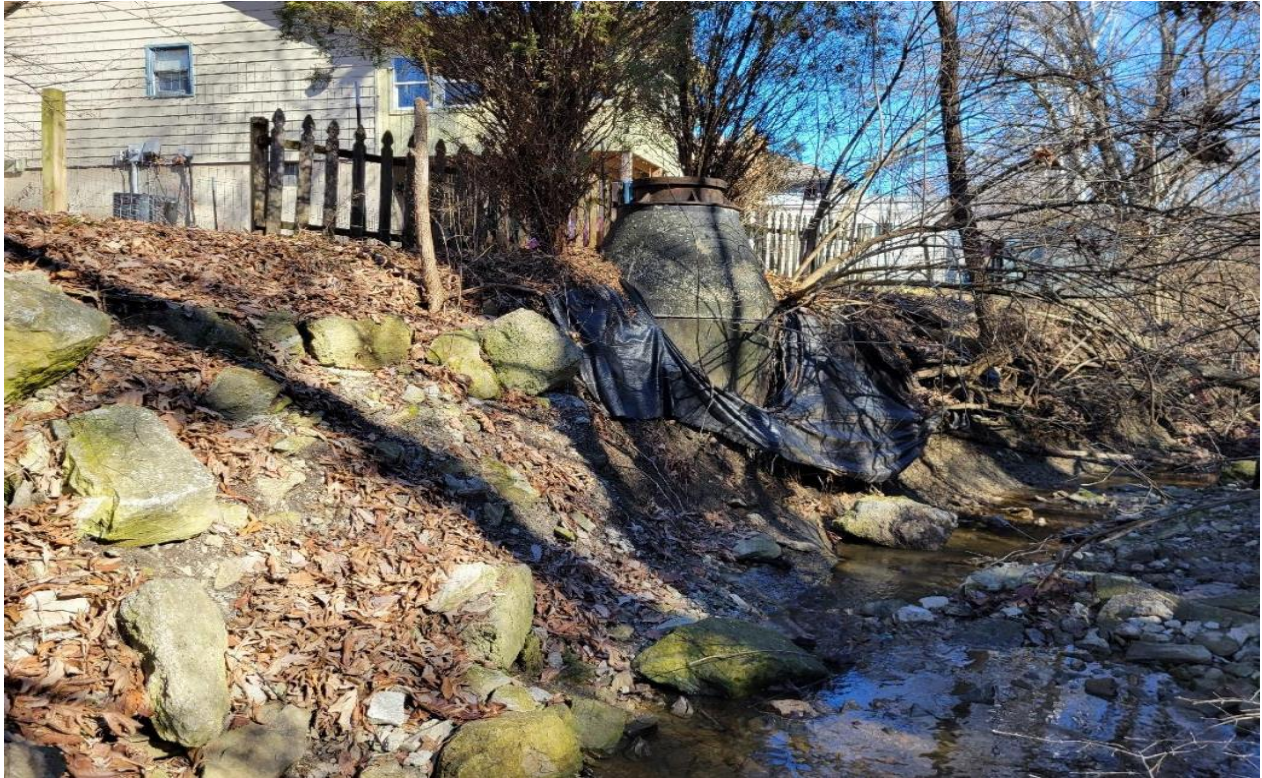
Figure 2-2. Observed Stream 1 Bank Erosion (Location ID: S1.17)
