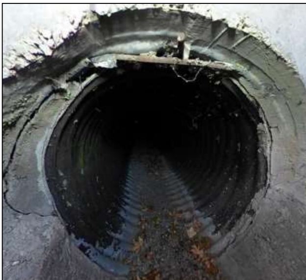
C11-10-1337: Rebar intruding through pipe seal
