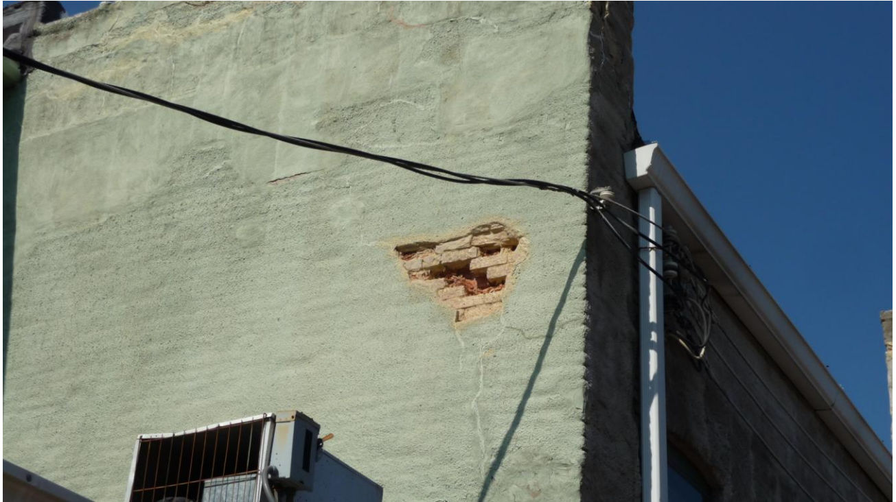
Physical Deterioration. Façade deterioration scattered throughout Redevelopment Area. Health and safety hazard from falling debris, also social liability (unattractive).
