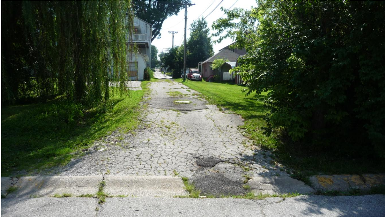
Physical Deterioration. Deteriorated alleyway pavement. Contributes to ill health, injury to pedestrians, bicycle and automobile traffic.
