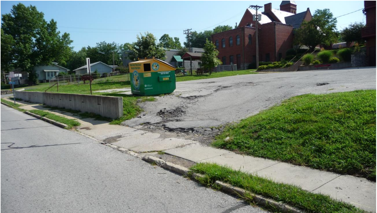
Physical Deterioration. Deteriorated surface parking pavement, curb & gutter. Social and economic liability as deterioration can lead to physical injury and private property damage (i.e. vehicular damage, flat tires, etc.)
