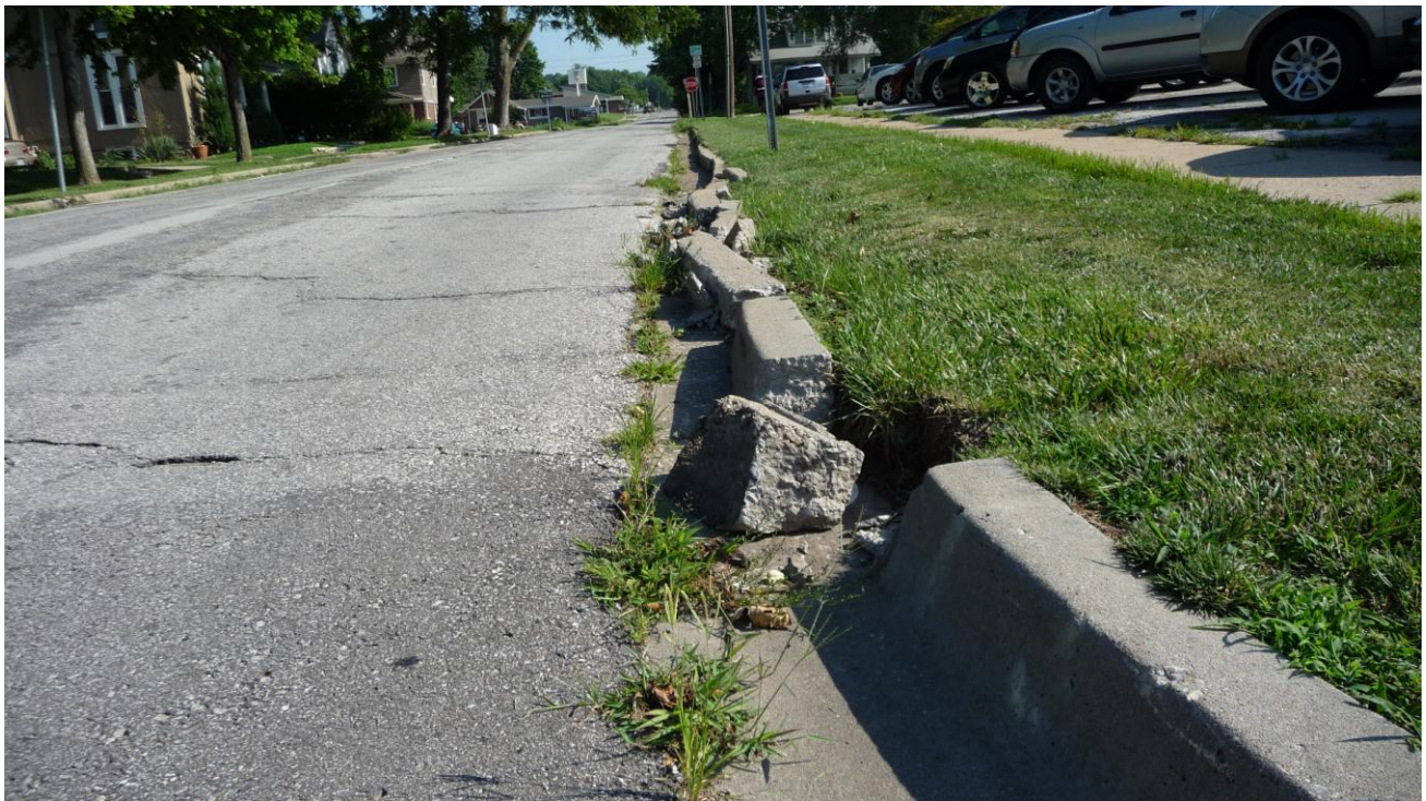
View typical deteriorated curbs & gutters. Present across much of Redevelopment Area. Contributes to ill health, injury to pedestrians, bicycle and automobile traffic.
