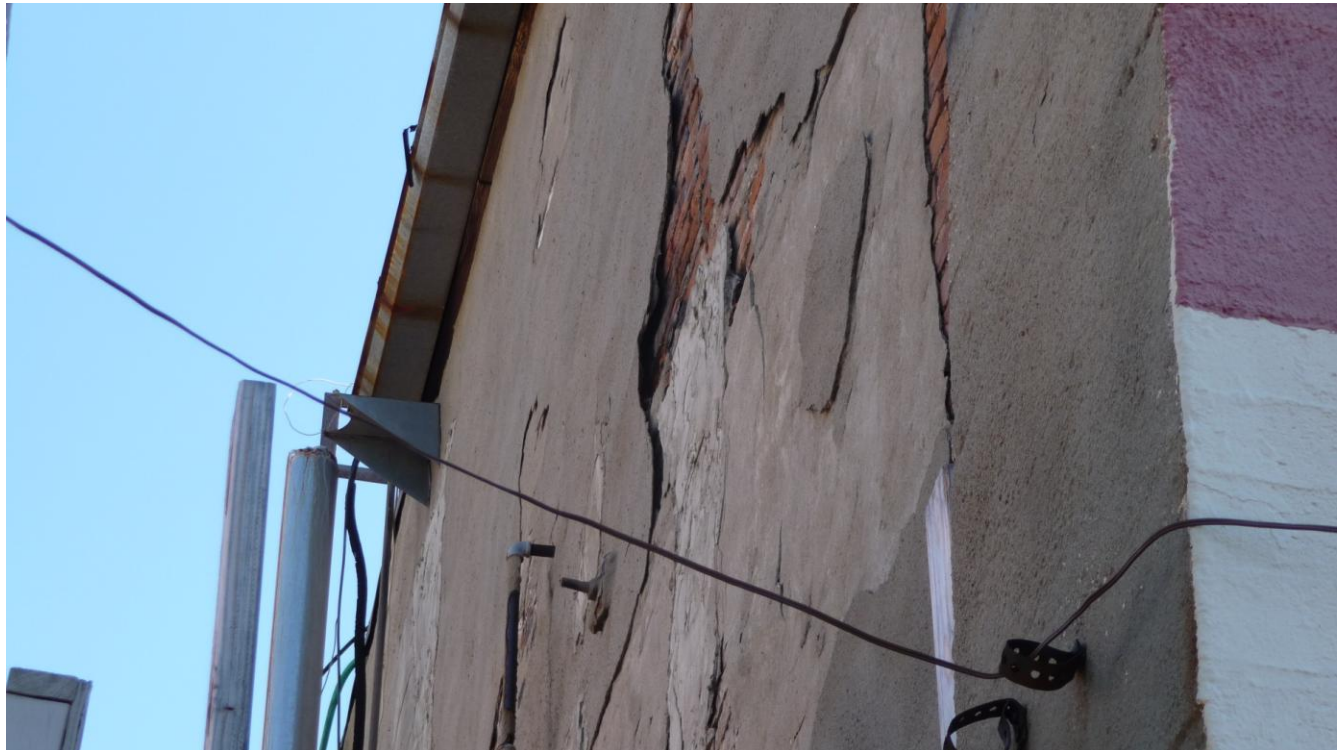
Physical deterioration of exterior building envelope. Exterior stucco system failing due to age and water infiltration. Health and safety hazard from falling debris, also social liability (unattractive).
