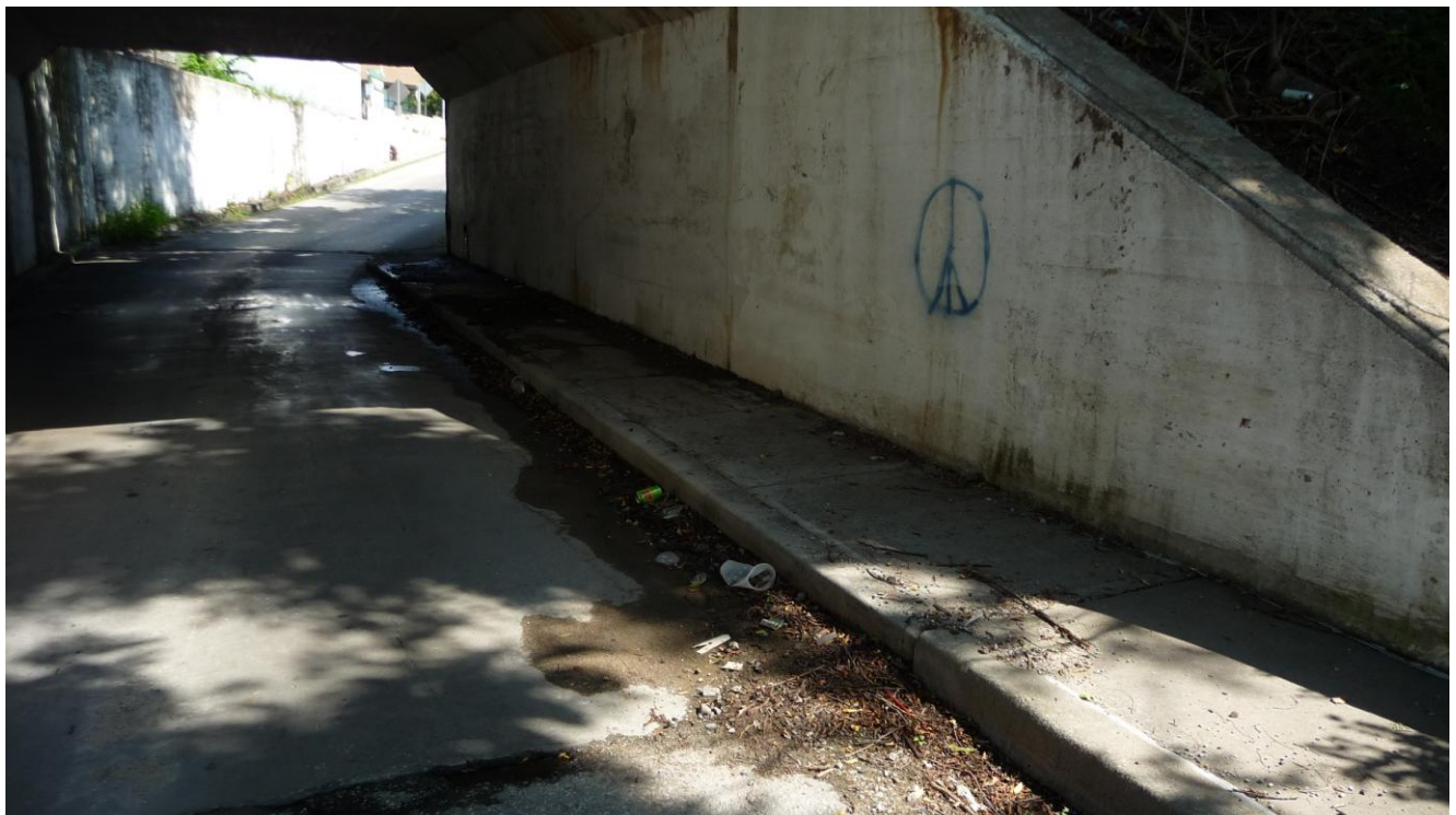
Outmoded Design. Note lack of visibility for on-coming traffic. Also crime-graffiti, and ill health, disease caused by trash and debris.
