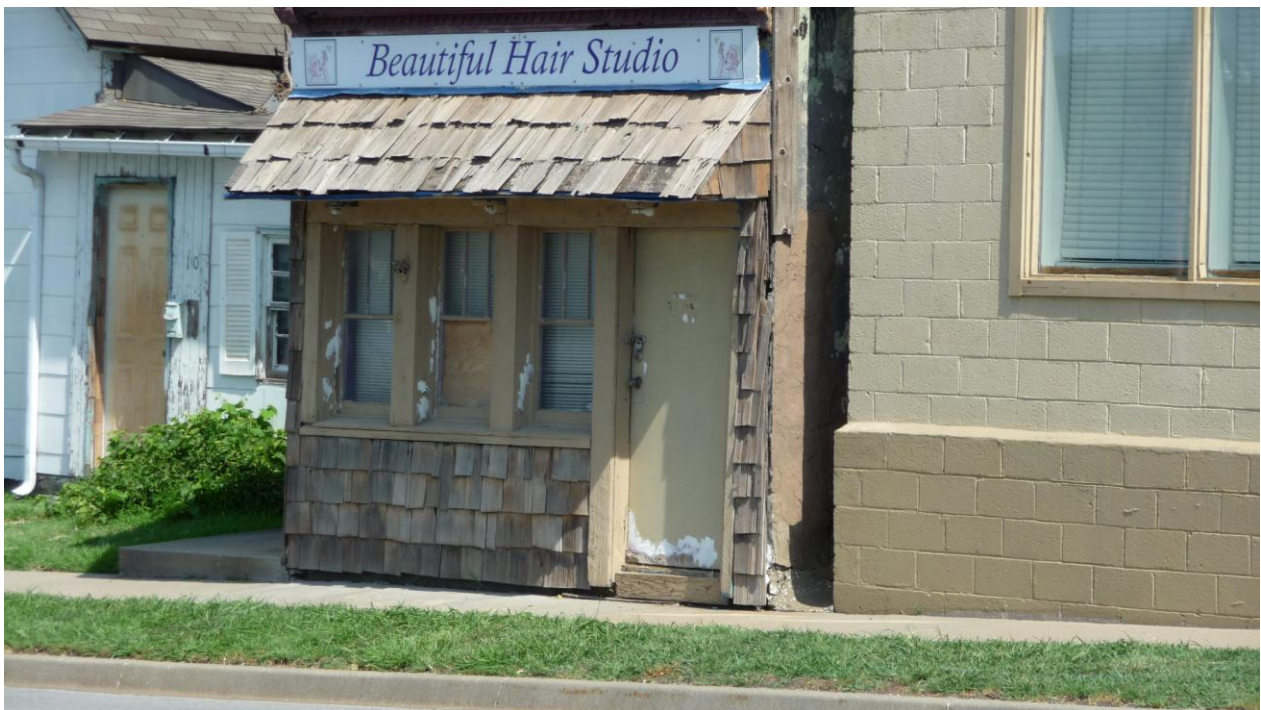
Physical Deterioration and outmoded design. Peeling paint, broken window, deteriorating façade elements of former hair salon. Also facility not ADA compliant.
