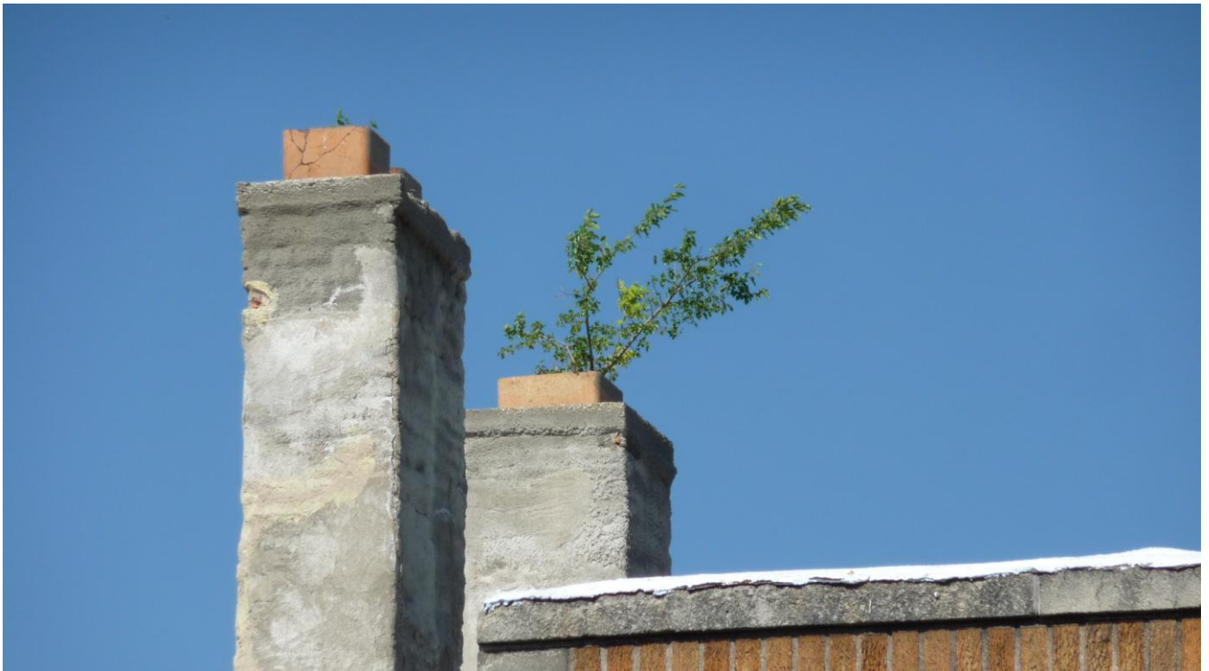
Deterioration. Vegetation growing from building exhaust chimney.
