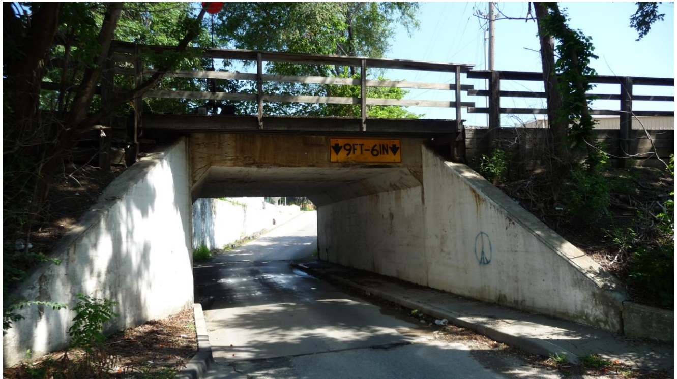
Obsolescence, deterioration and outmoded design. Single-lane, low clearance bridge on South Missouri Street.
