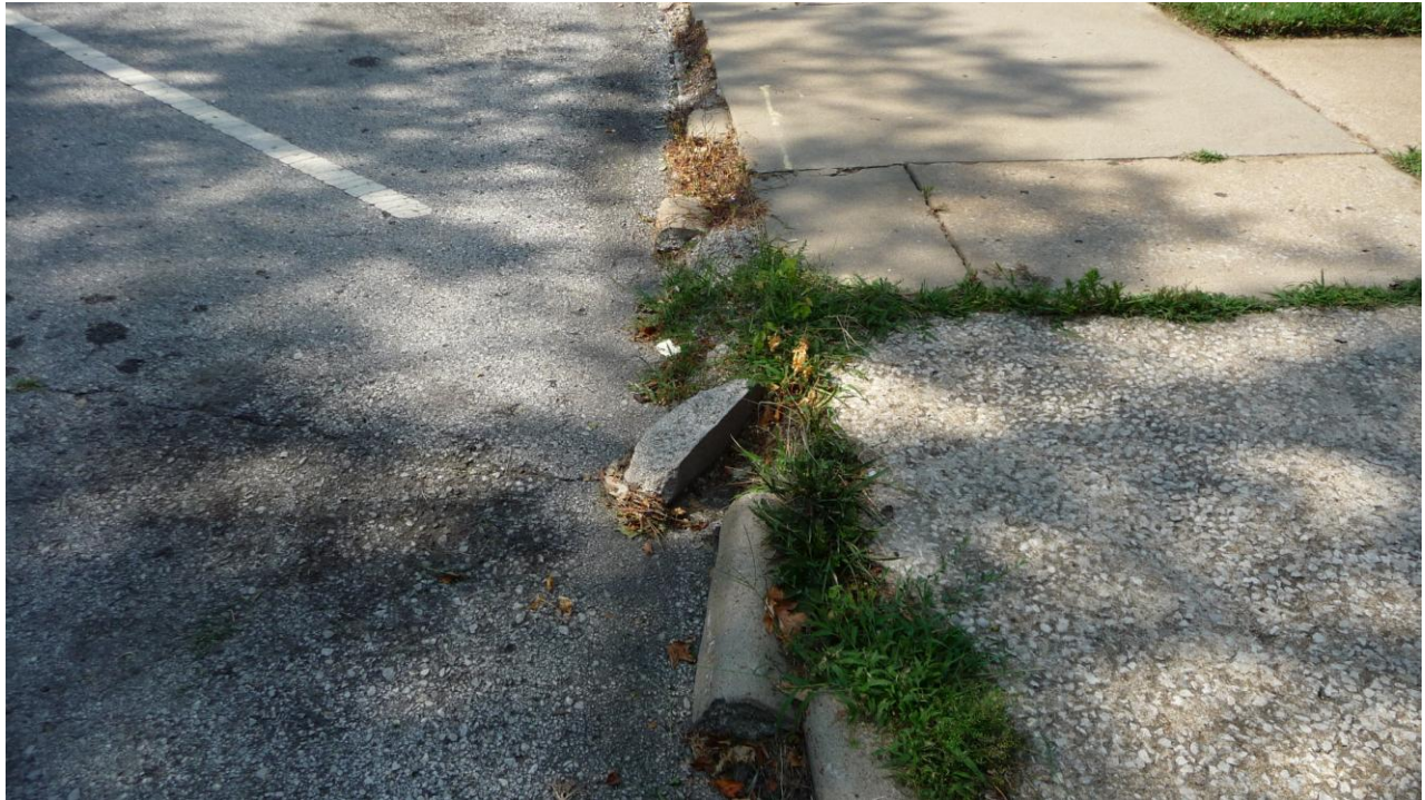
Physical Deterioration. Deteriorated curb & gutter infrastructure. Social and economic liability as deterioration can lead to physical injury and private property damage (i.e. vehicular damage, flat tires, etc.)
