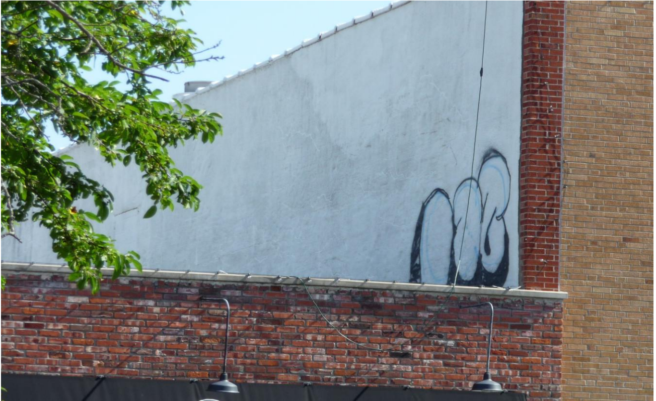
Deterioration, graffiti. Crime, ill health and potential injury from climbing structure to write graffiti.
