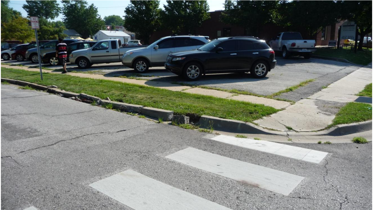
Physical Deterioration. Deteriorated curbs & gutters. Contributes to ill health, injury to pedestrians, bicycle and automobile traffic.
