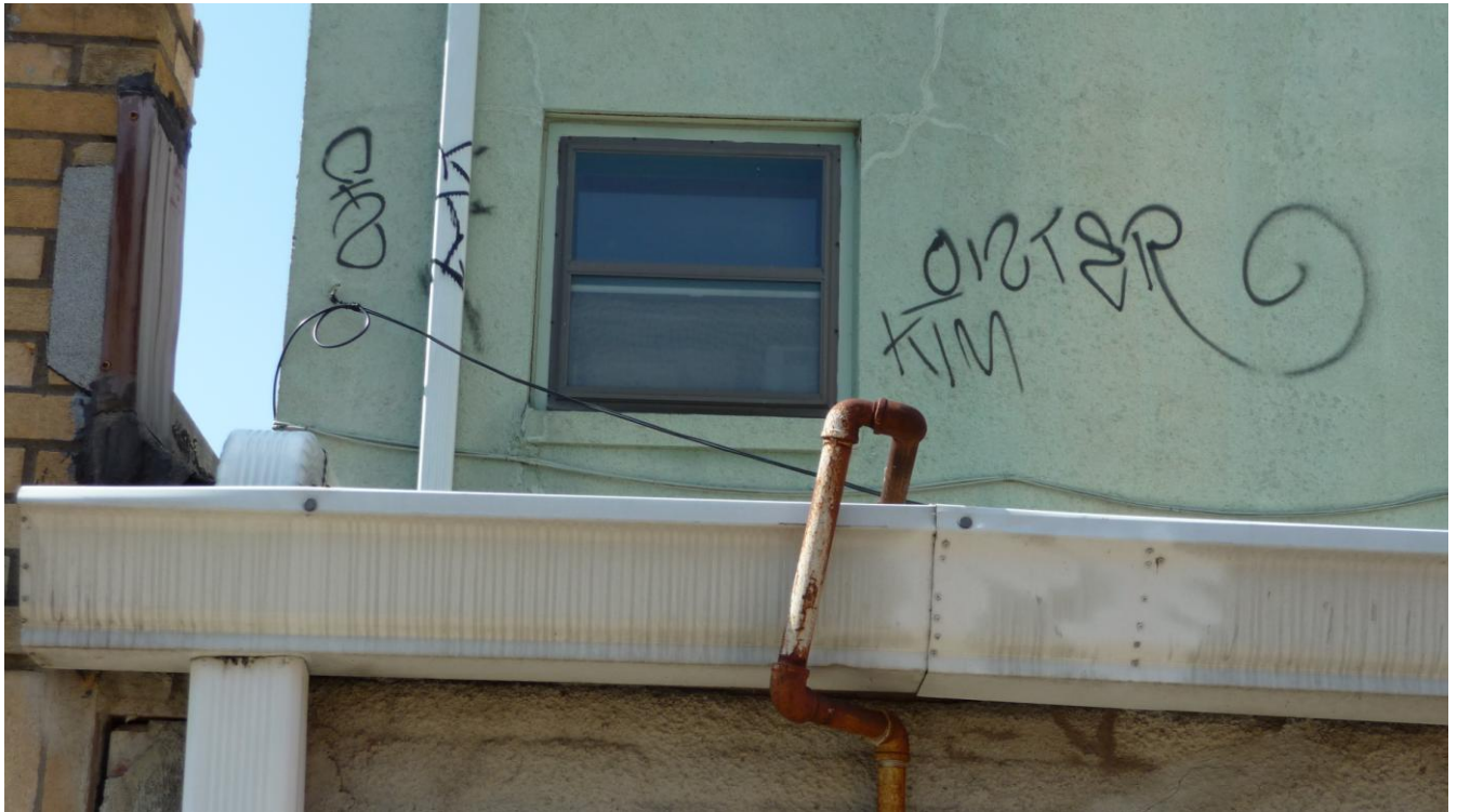
Deterioration, graffiti. Crime, ill health and potential injury from climbing structure to write graffiti.
