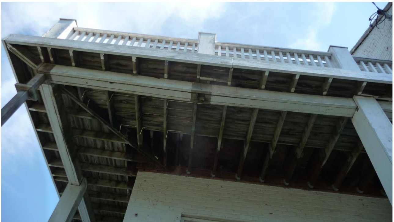
Physical Deterioration. Observable deck structure element removed with no reinforcing. Ill health due to the potential for life and safety issues.
