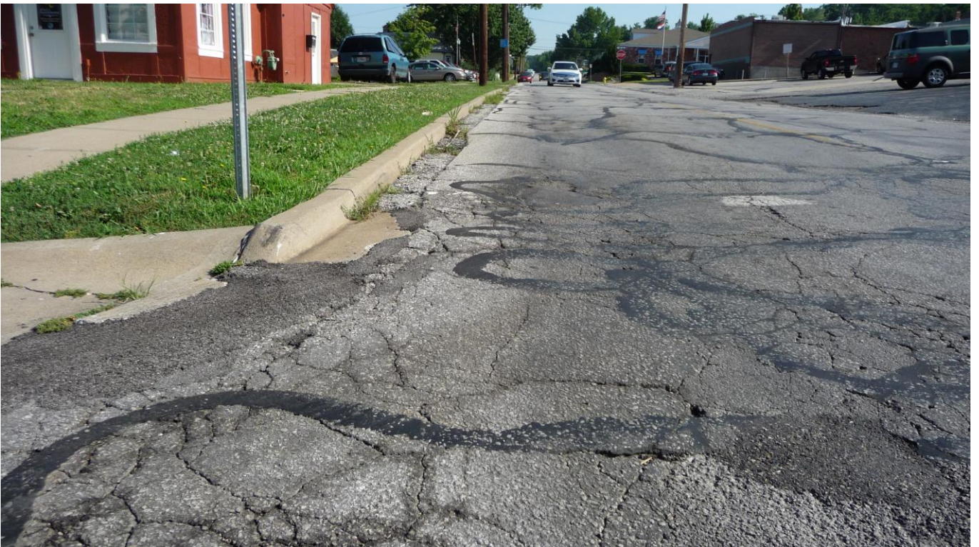
Physical Deterioration. Deteriorated infrastructure. Social and economic liability, unattractive public access reduces likelihood of reinvestment.
