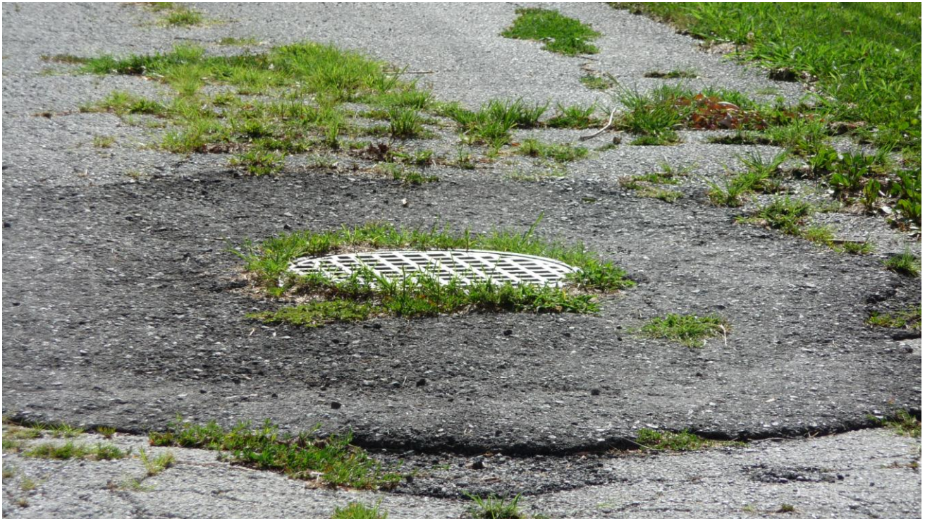
Deteriorated alleyway pavement. Contributes to ill health, injury to pedestrians, bicycle and automobile traffic.
