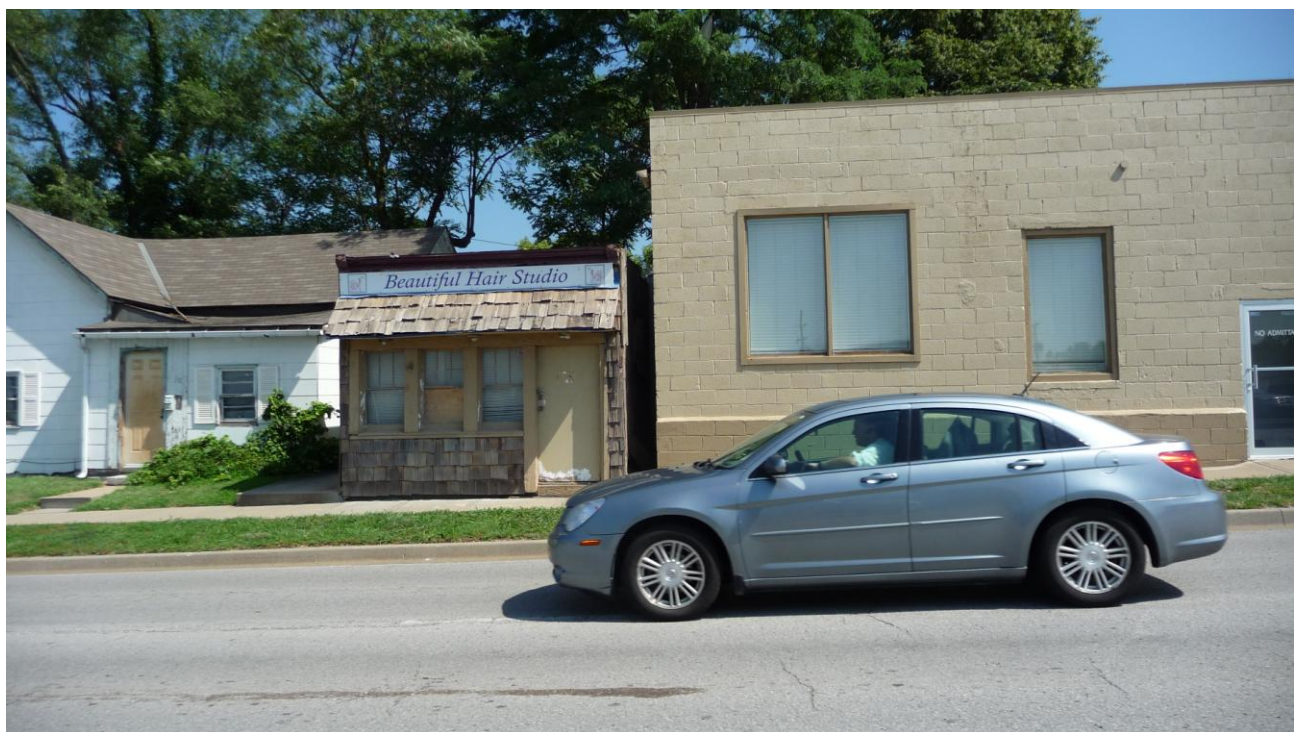
Physical Deterioration. 10 West Mill Street. Peeling paint, broken window, deteriorating façade elements.
